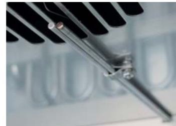
Multi-conductor temperature sensors
