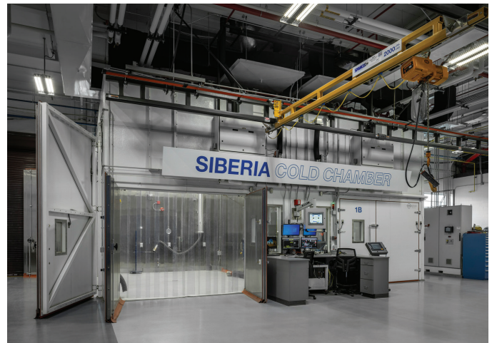
Climatic test chamber installed and integrated as part of applications lab renovation to expand engine manufacturer capabilities.
